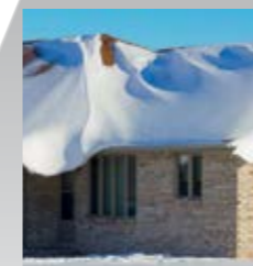
Unsuitable snow retention:
